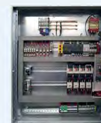
Pannello di controllo con PLC Control panel with PLC
