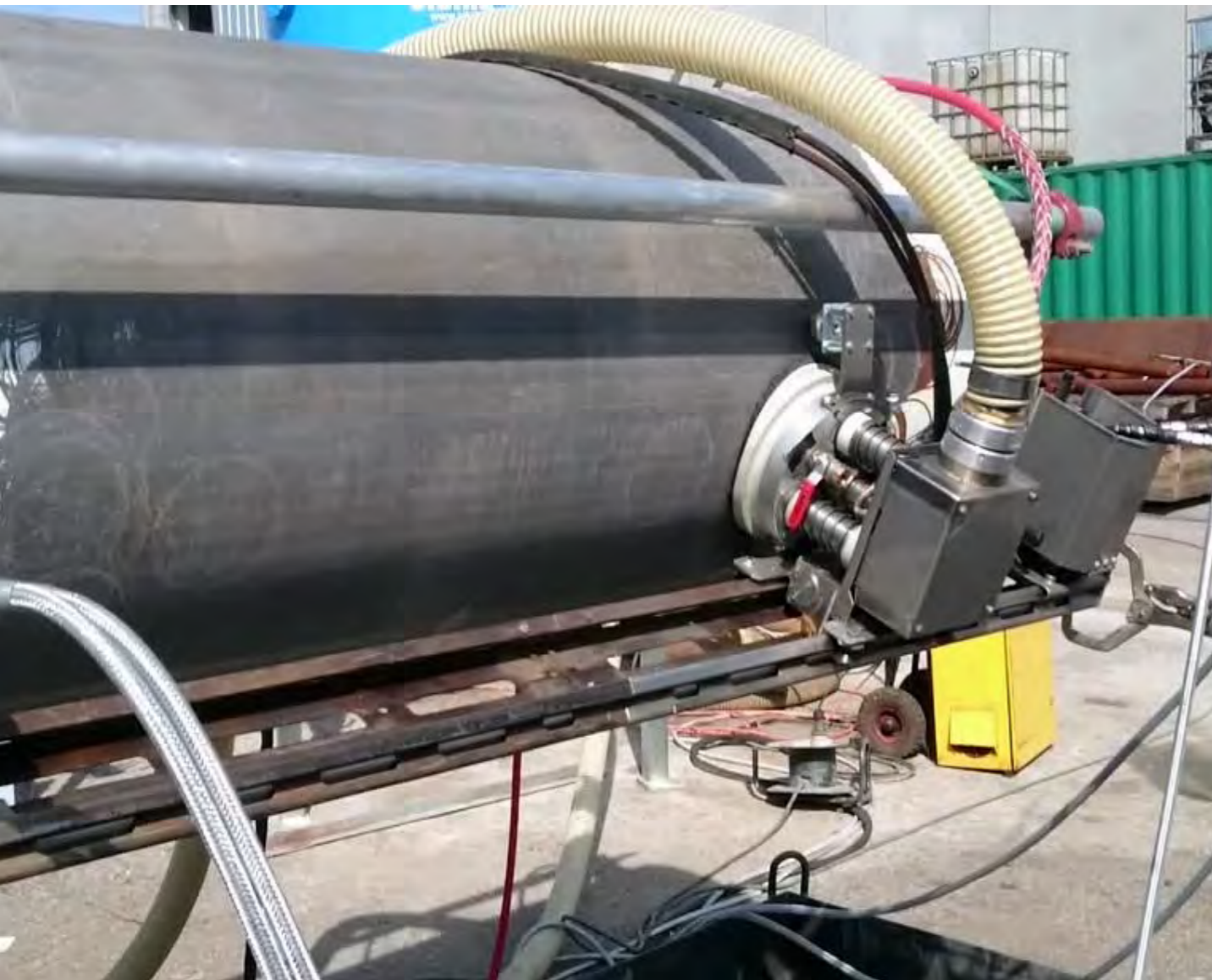
Nalta Jetframe 101, equipped with a rotor cradle and vacuum suction, used on a steel pipe for toxic paint removal.
