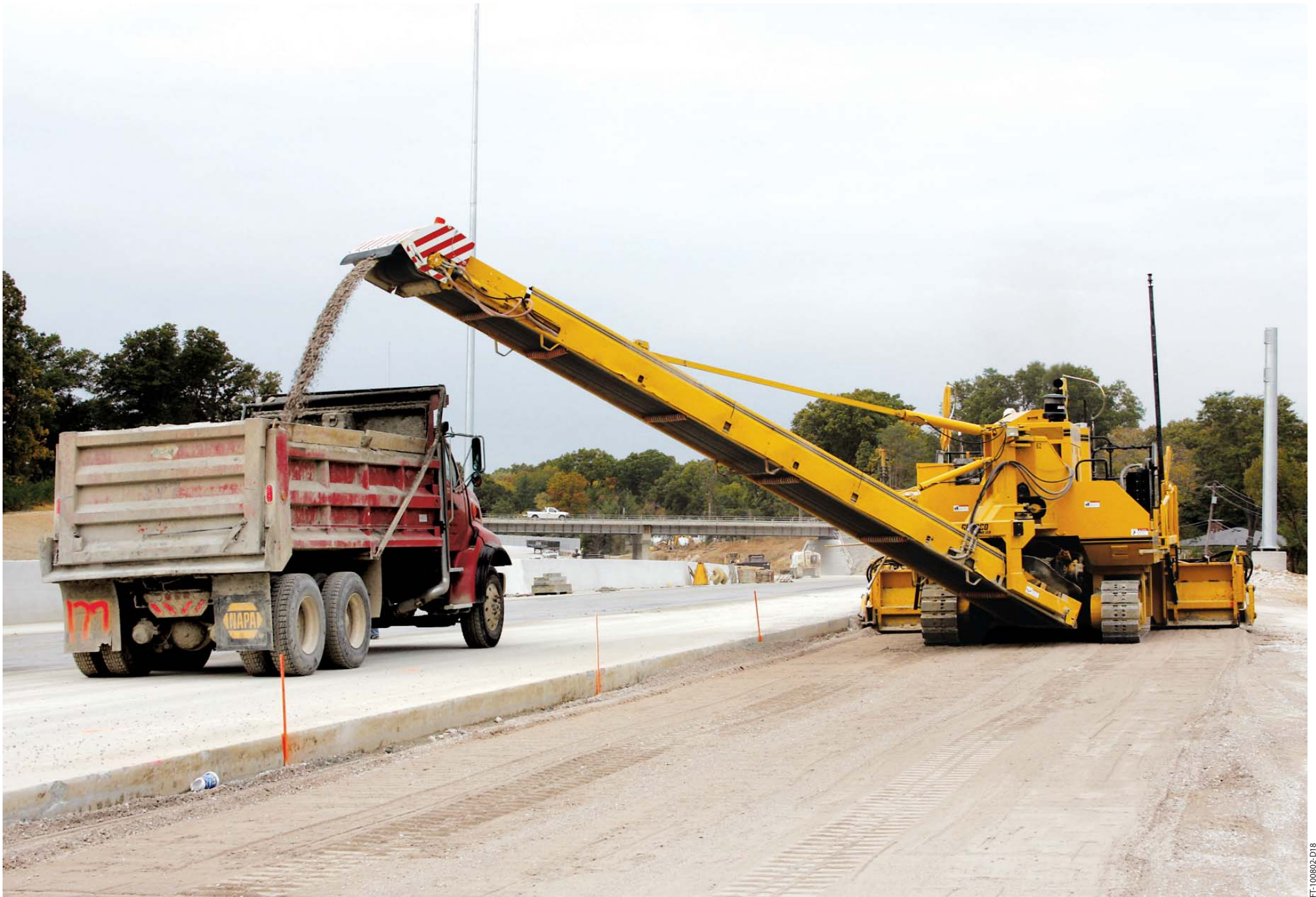
A GOMACO 9500 trims the grade and uses the conveyor to easily place the material into a haul unit for quick removal on an interstate project.
