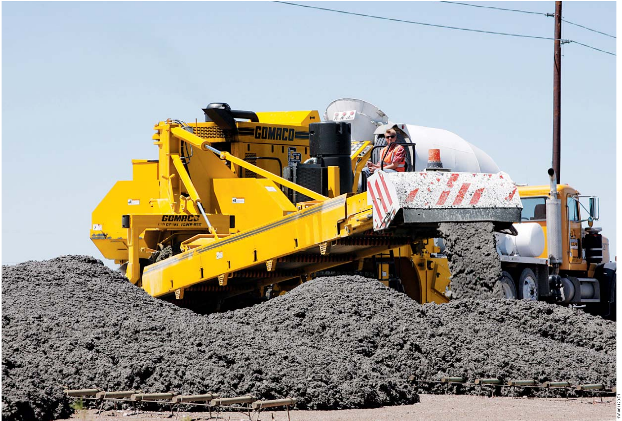
Placement of concrete with the 9500 is fast and accurate with the 35 foot (10.67 m) long conveyor.
