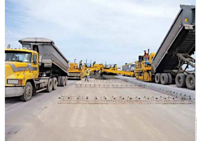
Two 9500 placers supply the concrete for the GOMACO paver on an airport runway.
