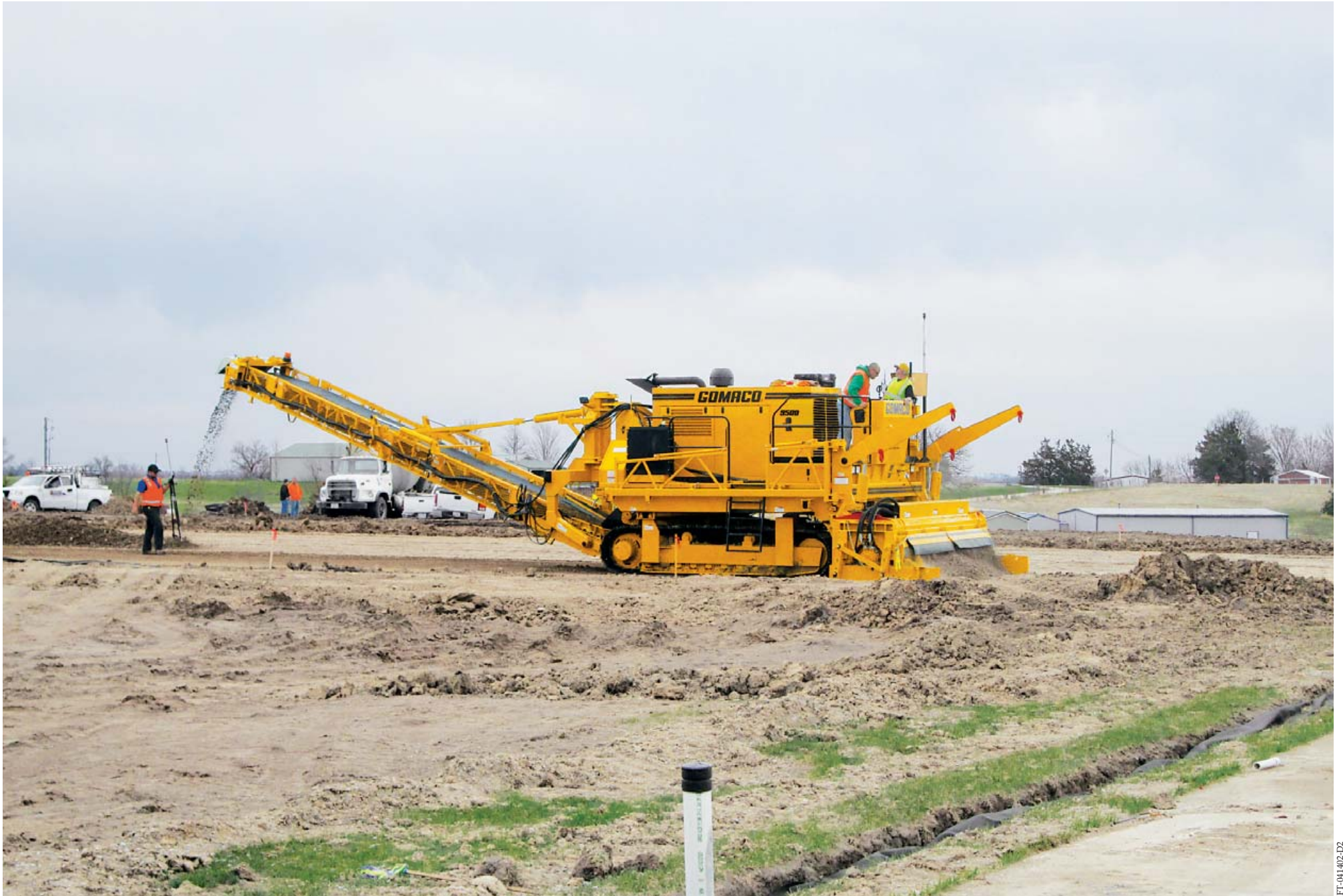
A GOMACO 9500 trimmer is equipped with a 14 foot (4.27 m) trimmerhead, G+ controls, and Leica Geosystems 3D machine guidance. The 9500 prepares the grade for 1000 feet (304.8 m) of airport runway and taxiway extensions.
