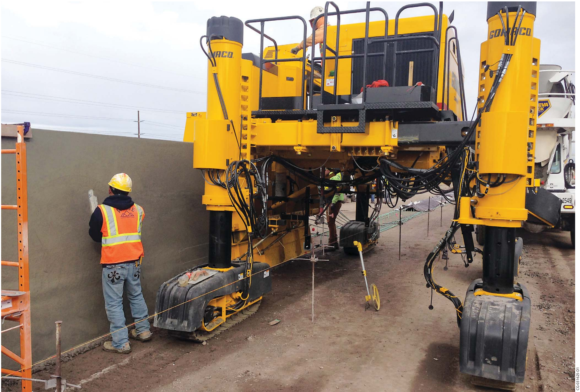
A seven-foot (2.13 m) tall barrier is being slipformed by the GOMACO Commander III four-track barrier package slipform paver.
