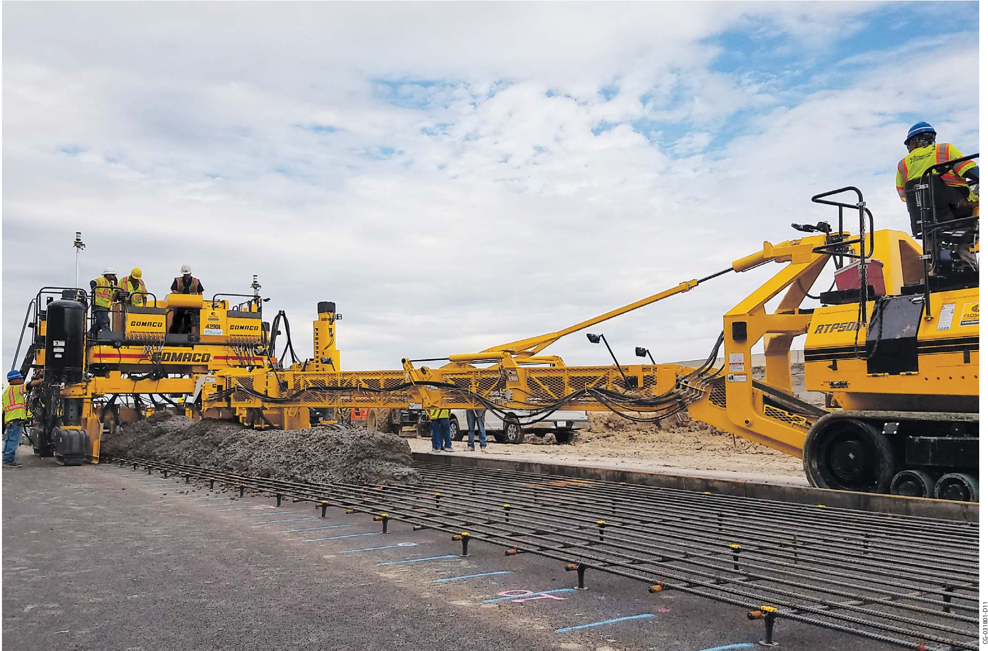
The GOMACO four-track Commander III slipforms a 12 foot (3.66 m) wide interstate ramp using 3D machine guidance. A GOMACO RTP-500 places the concrete over the steel reinforcement ahead of the Commander III.
