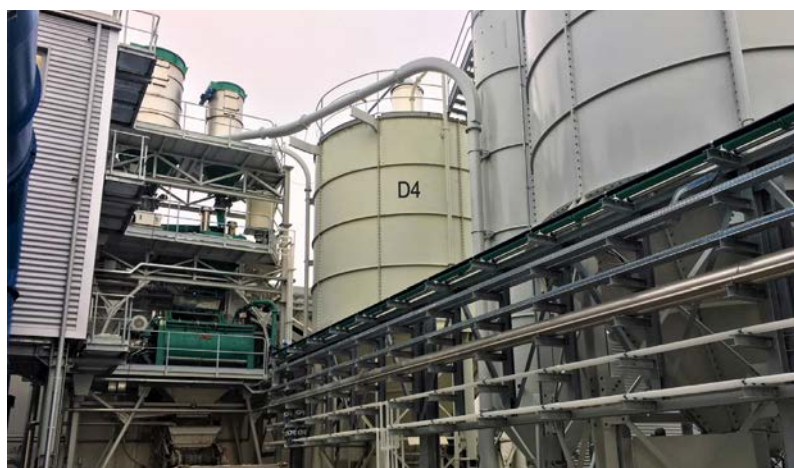
Foggia, Italy: Waste treatment plant
